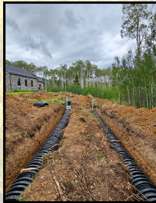
Chapel Septic System
